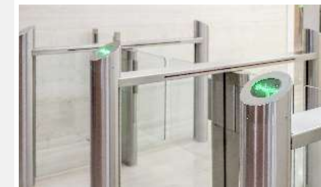
Access Controlled Lobby
